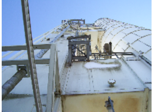
Figure 1: Ground View of Air Separation (ASU) & Argon side of Cold box
